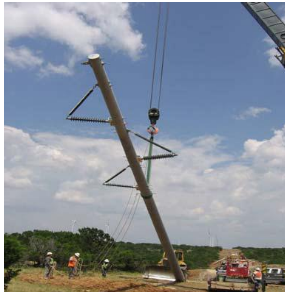
Figure 2-11: Typical Overhead Transmission Line Structures
