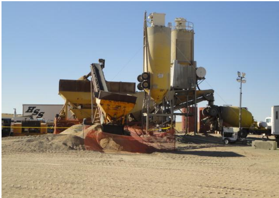
Figure 2-3: Typical Temporary Concrete Batch Plant
